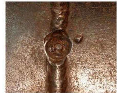
Example of Burn through
